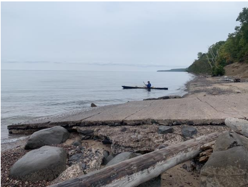
Figure 8. Agate Beach Boat Launch (currently in disrepair). Looking northeast.
